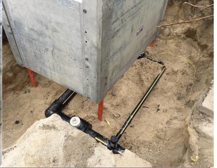
Unitil Gas Line Expansion Bypass Pipe & Valves @ South Side Parking Area 7-12-18 (1)
