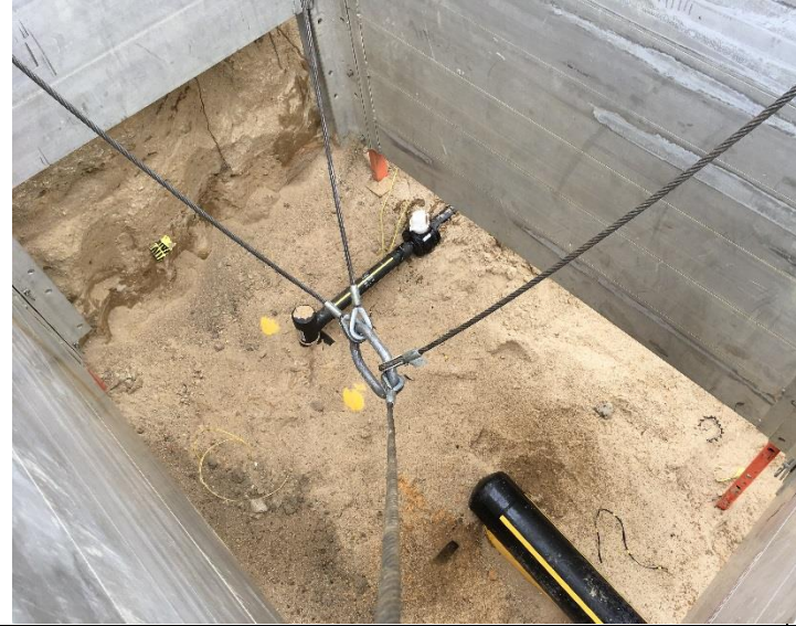
Unitil Gas Line Expansion Bypass Pipe & Valves @ South Side Parking Area 7-12-18 (2)
