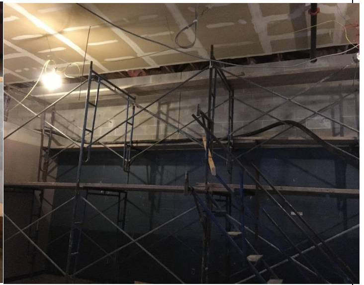
Rm.200 Grout Pump Line 7-11-18
