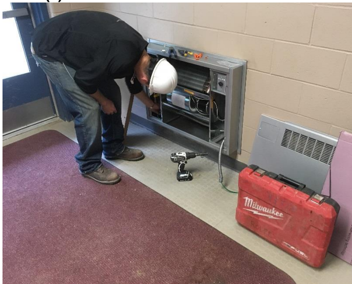
New Cabinet Unit Heater @ Stair-2 Entrance 9-26-18 (3)
